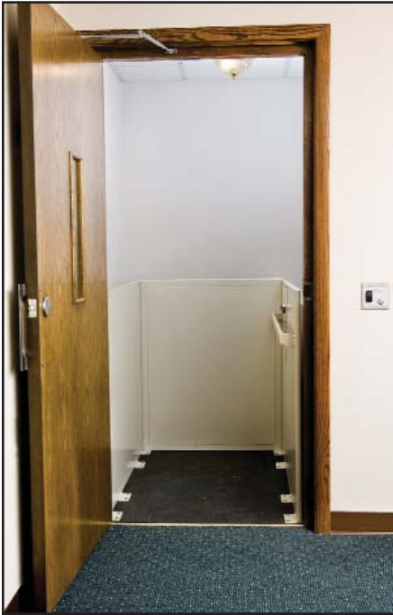
BC with runway enclosure built by others
